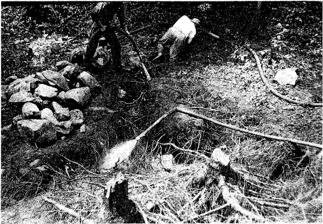
PLATE I. Following a single root. Cutting hose works fine material down to flushing hose. Trees are white oaks, Nos. 17 and 18.
