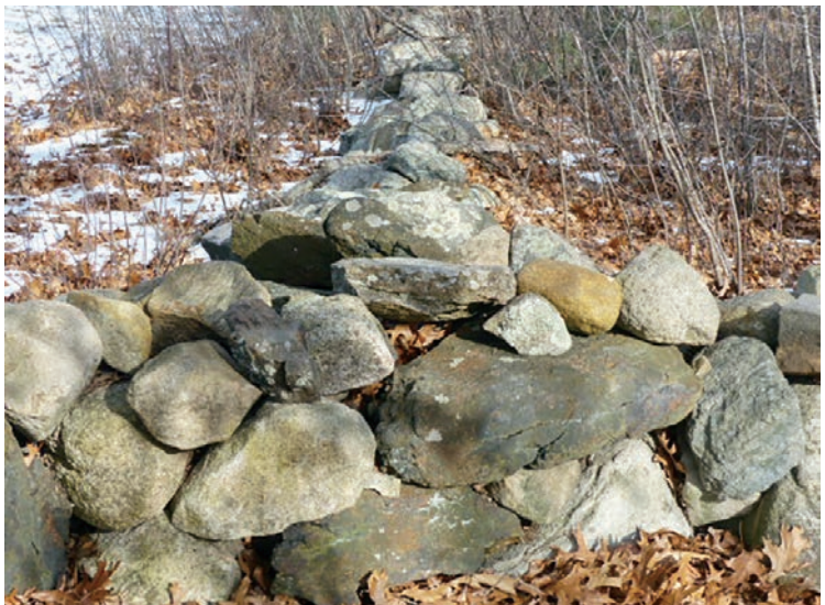
Figure 8 Diverse stone types illustrated at T-intersection. Gneiss, granite, one brown quartzite, and dark metasediment or metabasalt stones. USNPS Battle Rd., Lexington.
